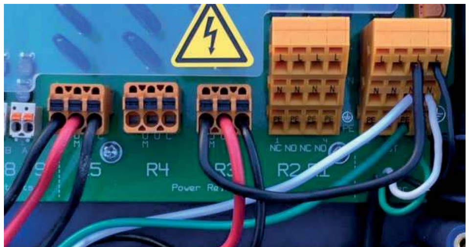
Figure 27 Motor Operated Valves wired to R3 and R5
