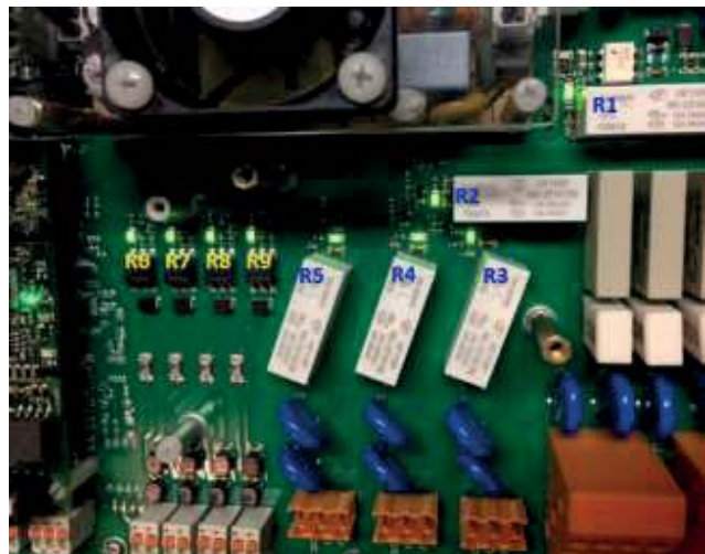
Figure 12 Internal Relay Indicator LEDs
