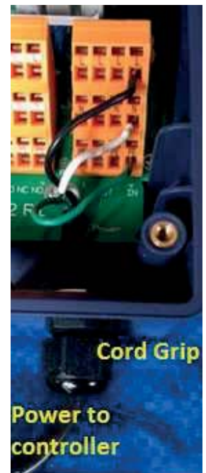
Figure 20 Factory installed Power
