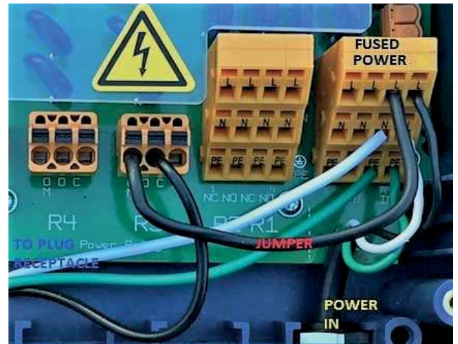
Figure 25 Wiring R3 using on-board fused power
