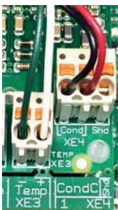
Figure 43 Four Wire Condensate Probe On XE2
